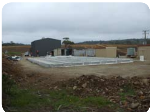
The Water Treatment Plant being prepared onsite.
