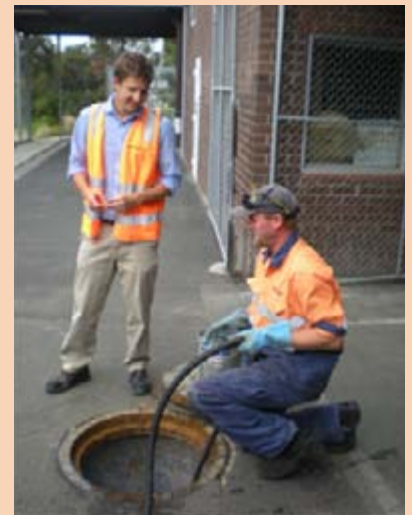
Wastewater Source Management Officer Nigel McCormick (standing) examining the condition of a manhole with a Southern Water colleague.
